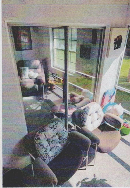
Unprotected glazed entry door
